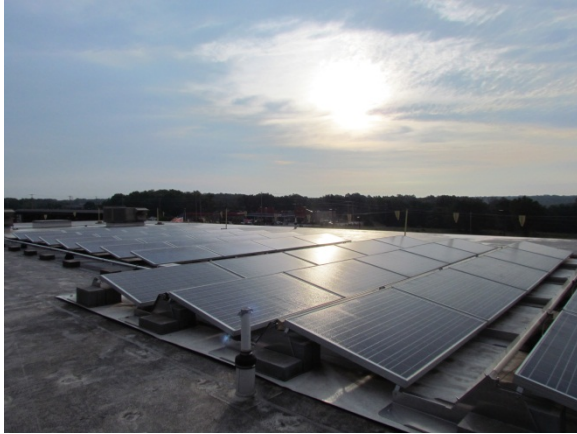
Figure 1 - 10 kW solar system installed as part of the Solar One Pilot Program. Photo courtesy of Columbia Water and Light
