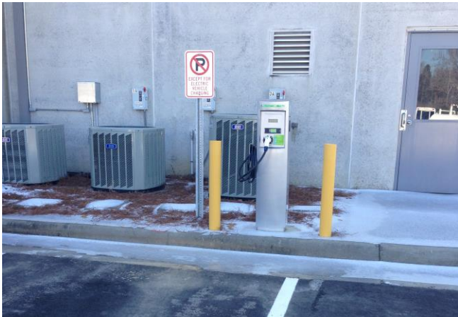
A newly installed Level 2 Electric Vehicle Charger in the City of Concord.
