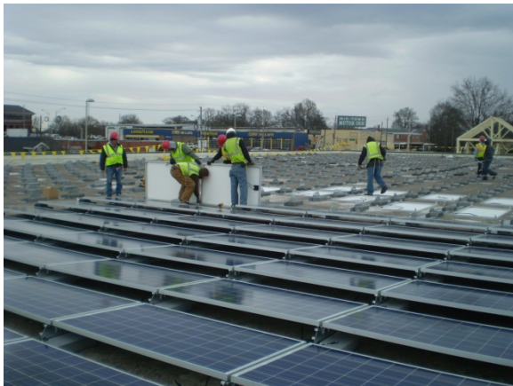
Figure 1 - NARENCO crew members work over the holidays and through inclement weather to ensure installation is completed by the end of the year. Photo courtesy of NARENCO.
