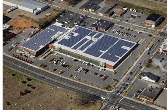
Figure 2- Completed rooftop solar installation on York Chester Plaza building. Photo courtesy of NARENCO.
