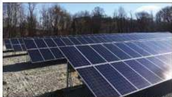
SOLAR GARDEN —On the hill above and behind the Blue Ridge Energy office in Sparta sits an array of solar panels that will power homes and businesses in Alleghany County.
